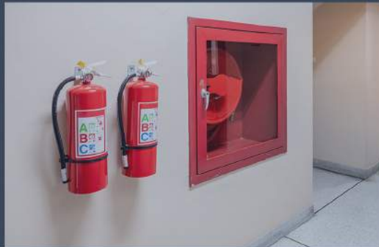
Fire fighting equipment as per norms
